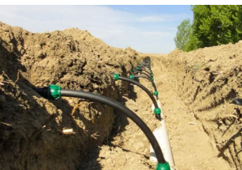
Underground drip irrigation.
